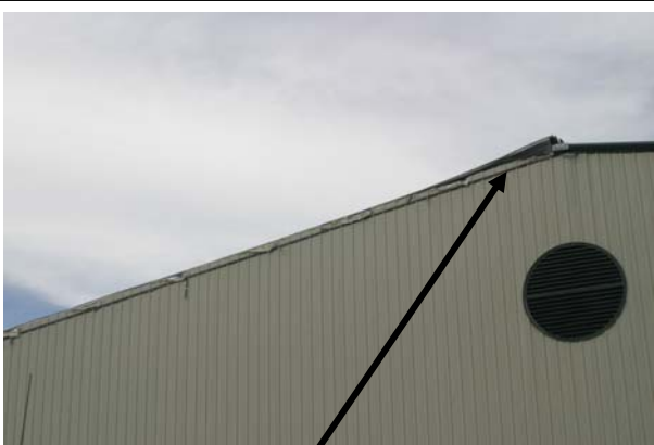
Leading edge failures lead to progressive peeling of the roof membrane.
