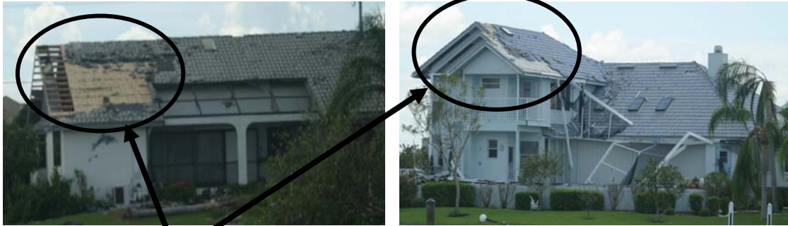
Classical damage pattern to gable end roofing material.
