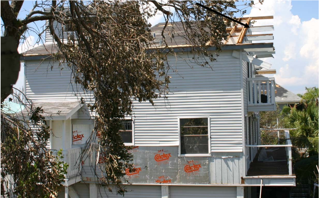
Progressive sheathing failure induced by failure of large overhang.
