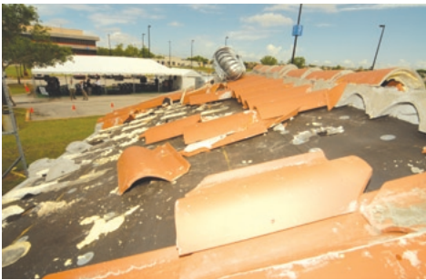
Roof damage after testing at 130mph
